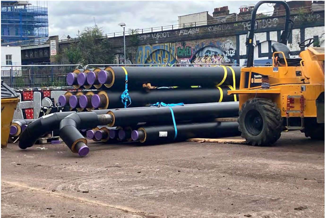
District Heat Network pipes
